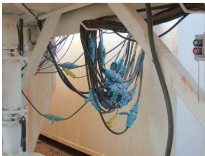
Multiple decontactors located throughout a drilling rig allow for safer and easier control of electrical power during rig moves (photo from Saber).
